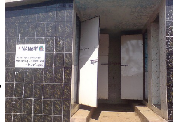
Clean ecosan public toilet
